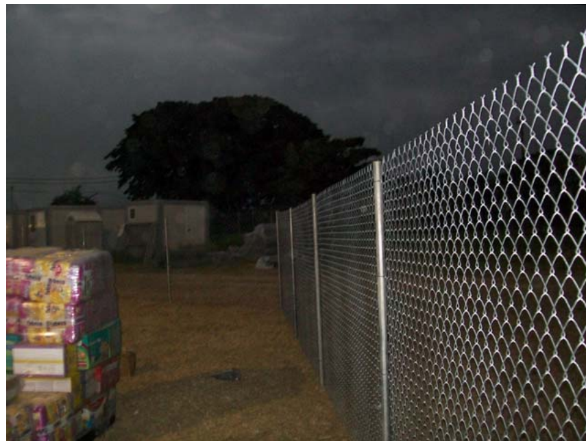
Carlson Fence and Master Halco provided labor and materials to help secure the hospital.
